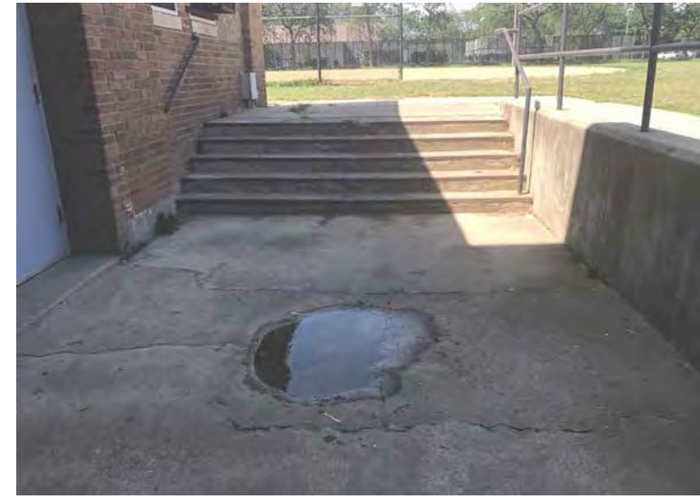
EXISTING PONDING AT DRAINS
