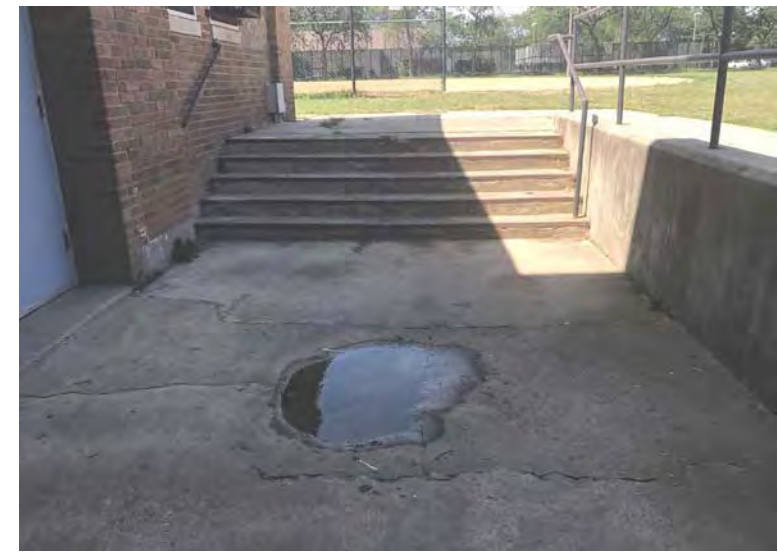
EXISTING PONDING AT DRAINS
