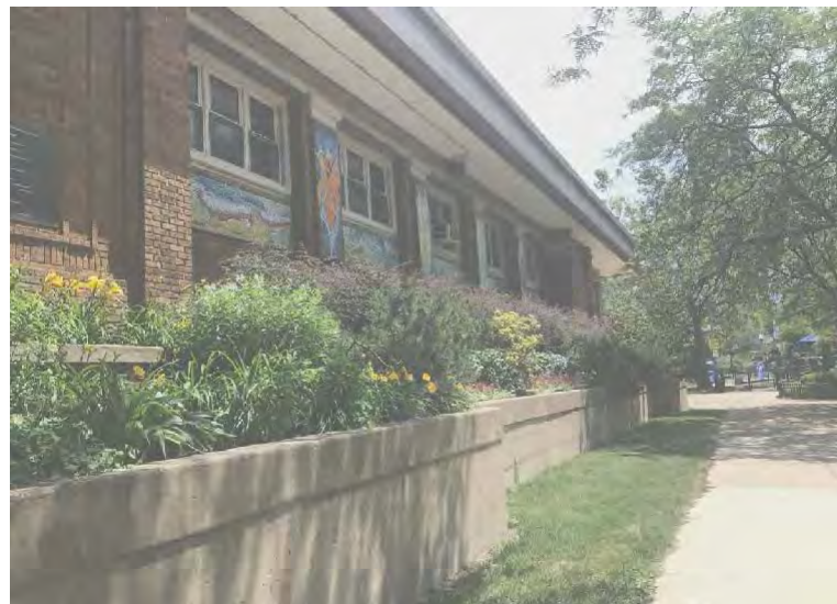
EXISTING LEAKING PLANTER
