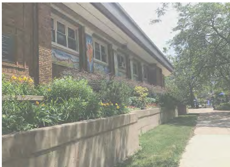
EXISTING LEAKING PLANTER
