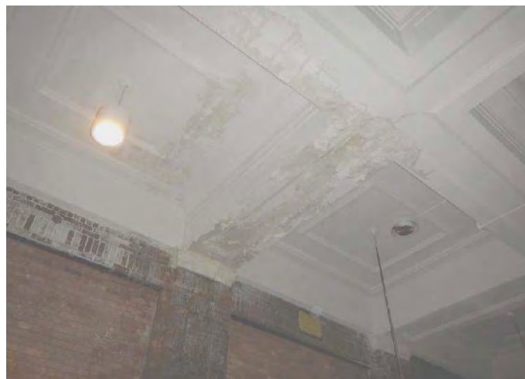
EXISTING MULTI-PURPOSE ROOM WATER DAMAGE
