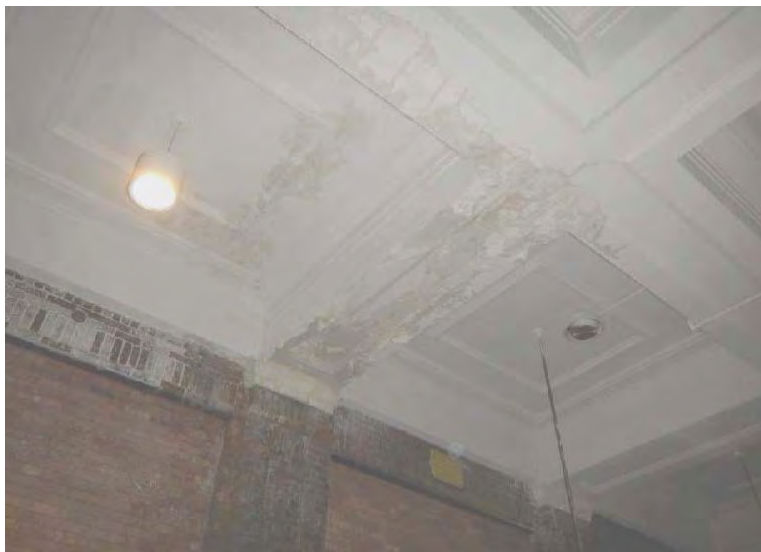
EXISTING MULTI-PURPOSE ROOM WATER DAMAGE
